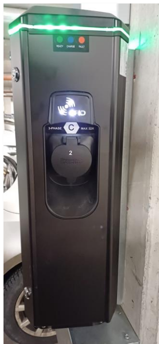
Figure 14: Electric vehicle charging unit installed at NSAI headquarters, Santry, Dublin
