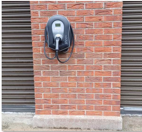
Figure 13: Electric vehicle charging unit installed at Galway Regional Office
