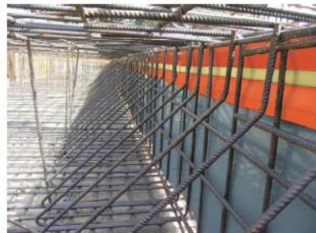
2. Crack induced joints
