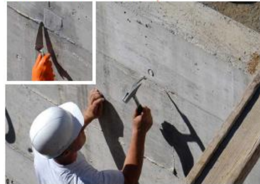
4. Formwork tie-bolt holes
