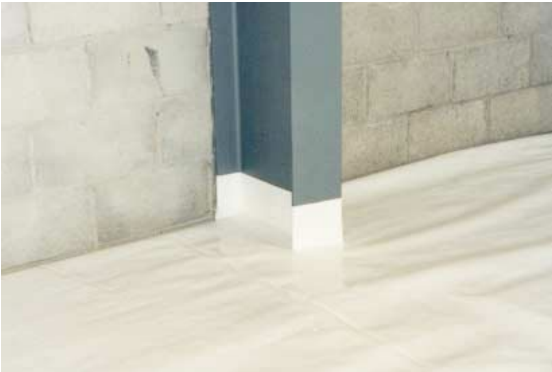
Fig 3: Detail showing structural steel stanchion with penetration seal
