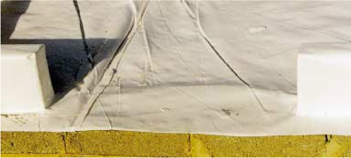
Fig 1A: Factory sealed fusion weld joint and wrap around radon protection detail on rising wall at external door opening
