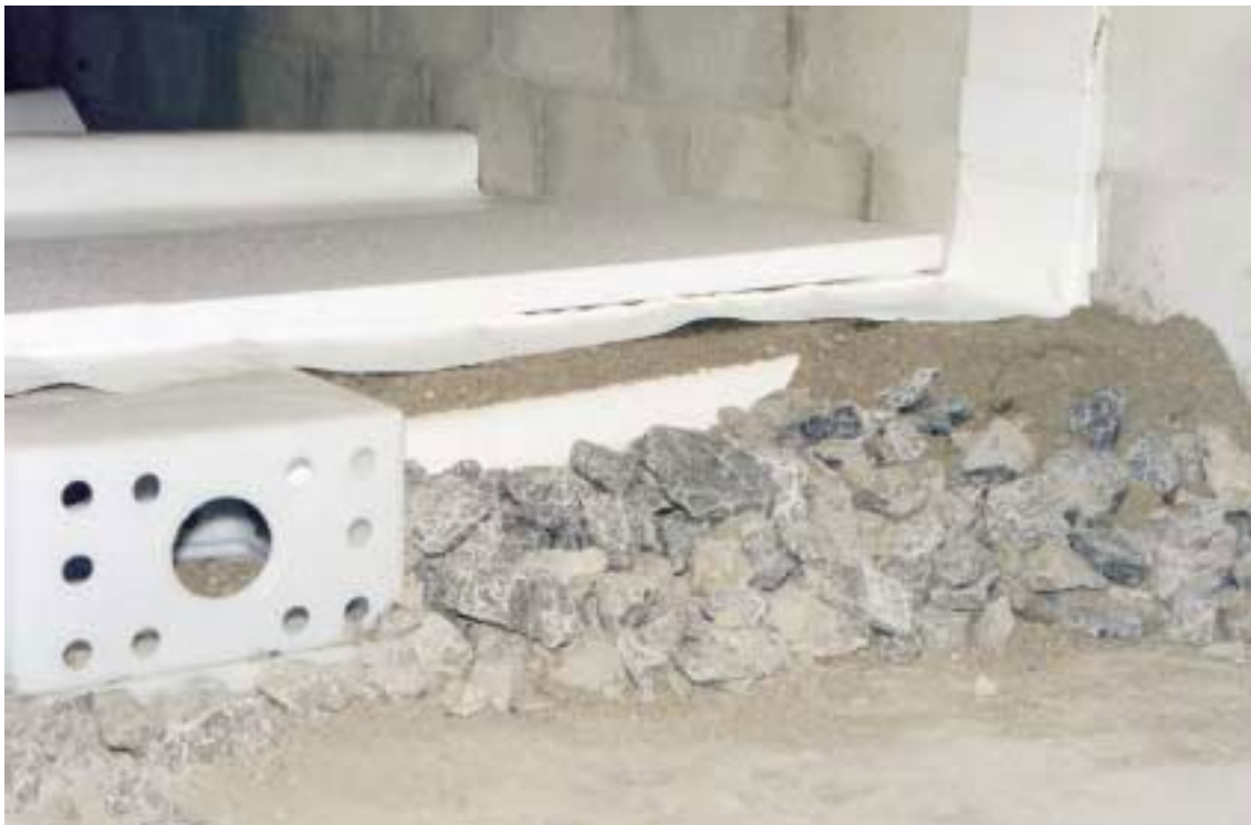
Fig 5: Section through a sub-floor showing the installation of a radon collection sump with proprietary white vent pipe system
